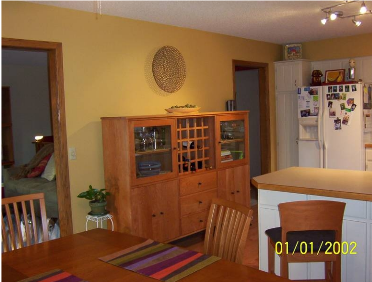
Figure 11: Perspective 1 showing the existing interior bearing wall separating the kitchen from the living room
