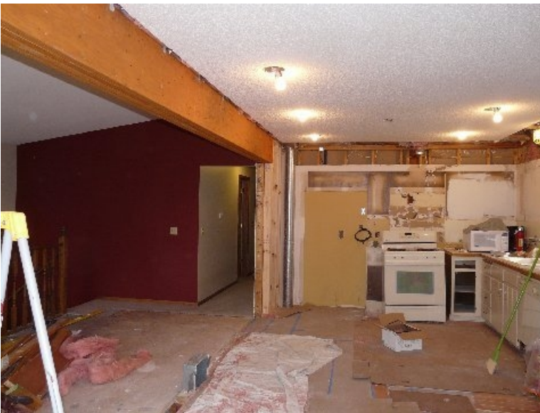
Figure 12: Perspective 1 showing the bearing wall removed and the new LVL beam installed
