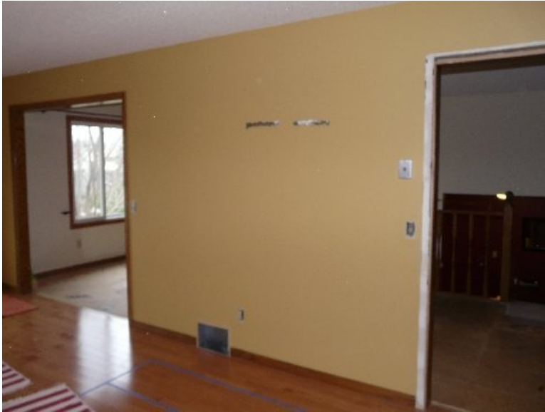
Figure 14: Perspective 2 showing the existing interior bearing wall separating the kitchen from the living room
